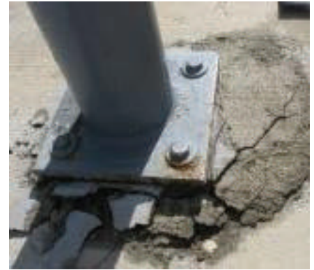
BOLLARD HIT BY SUBCONTRACTOR VEHICLE
